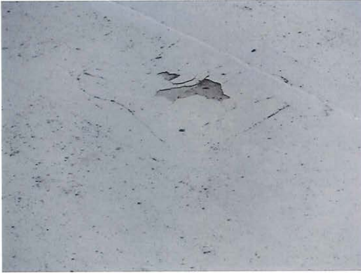
40) Spot coating failure on the roof inside the handrail.
