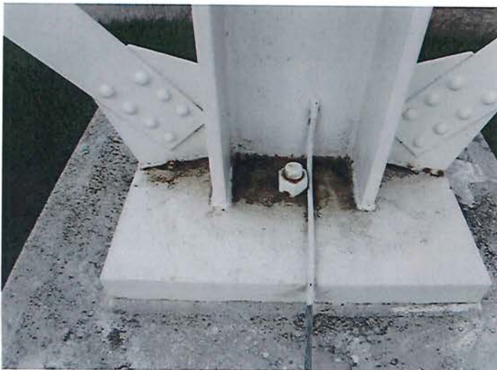
9) Typical anchor bolt is in good condition. There are minor spot coating failures on the baseplates.
