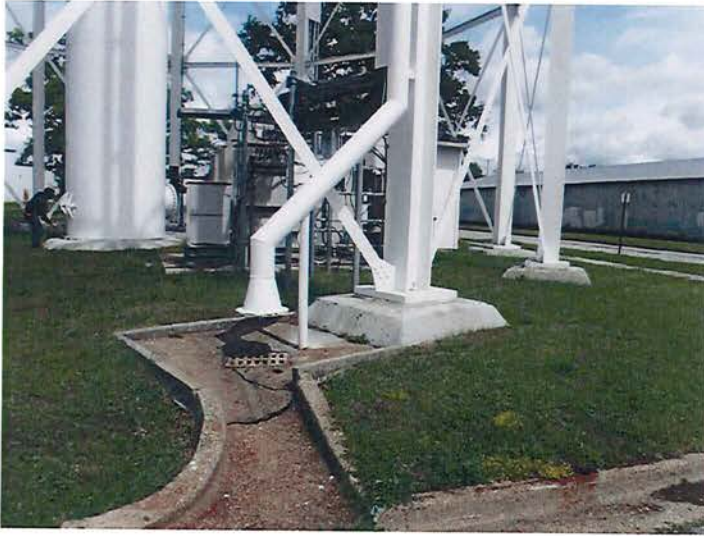
10) The overflow pipe discharges to a concrete catch basin.
