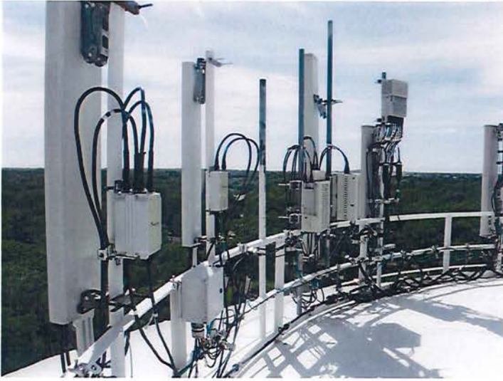
37) The roof handrail is in good condition and is being used for antenna mounting.
