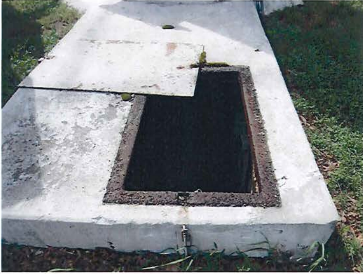
55) Hatch to the pit next to the riser.
