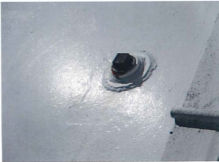
33) Typical rigging coupling on the roof.
