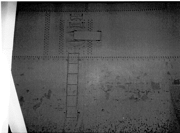
48) The ladder from the sidewall manway to the bowl is in good condition.
