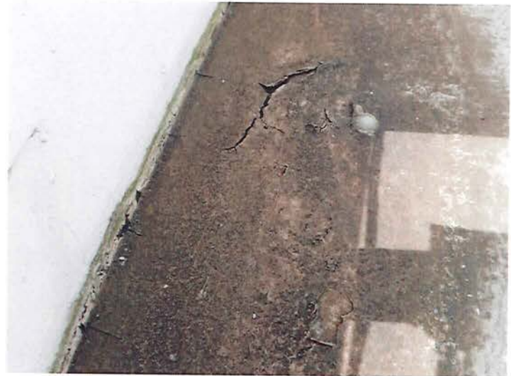
26) Spot coating failures on the top of the balcony.
