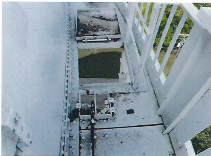
24) Balcony ladder opening with hinged cover.
