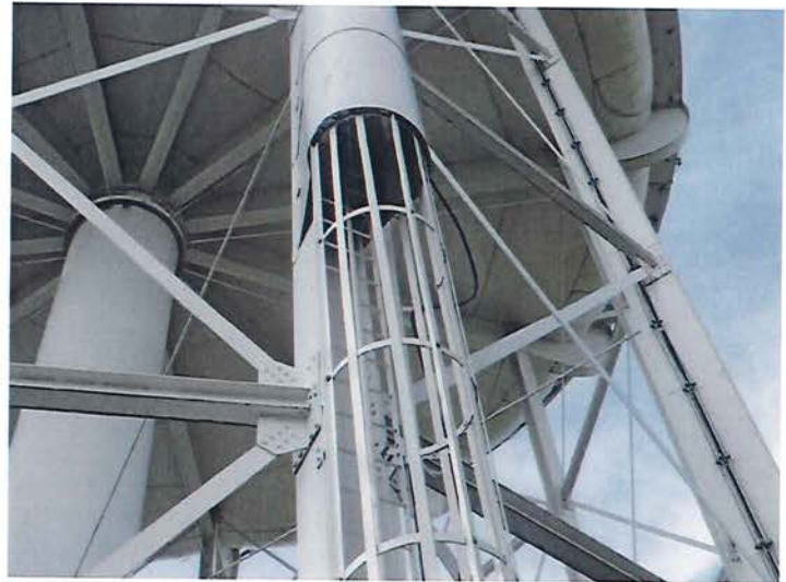
14) The leg ladder is caged and equipped with a rail-type fall prevention device.
