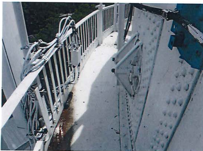
27) Dirt on the balcony is evidence of water pooling.
