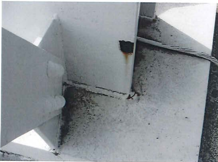
12) Spot coating failure on a leg.
