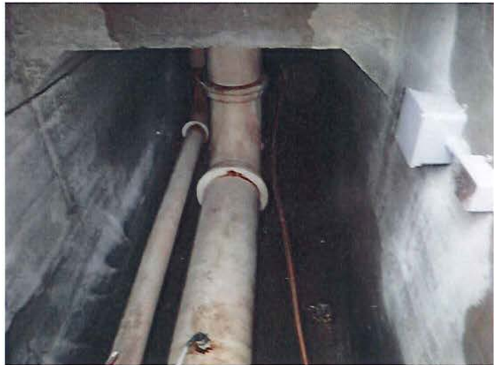
56) The coating on the piping is in fair condition with some minor coating failures.
