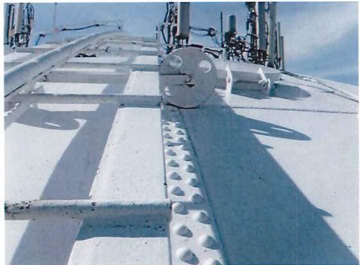
32) Sidewall/roof ladder and wet interior roof hatch.
