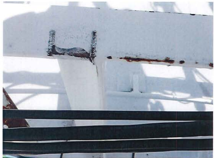
38) Spot coating failures on the roof handrail.
