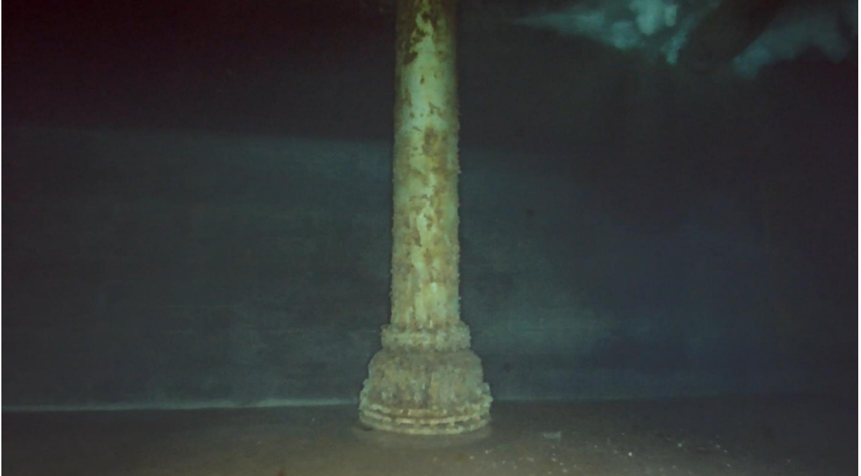
BACKWASH PUMP NO. 3 SUCTION LINE AND FOOT VALVE
