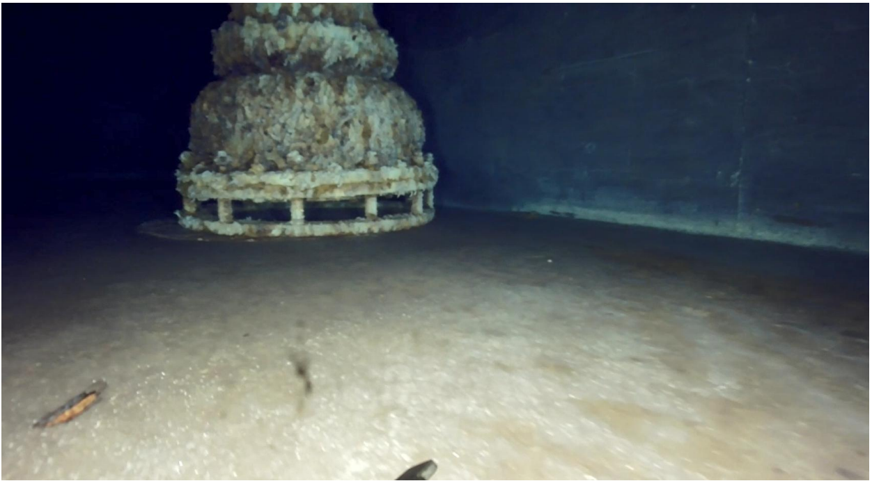
BACKWASH PUMP NO. 2 FOOT VALVE
