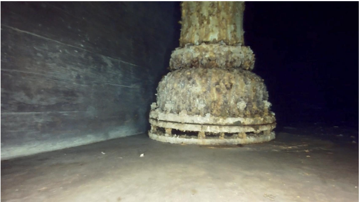
BACKWASH PUMP NO. 3 FOOT VALVE
