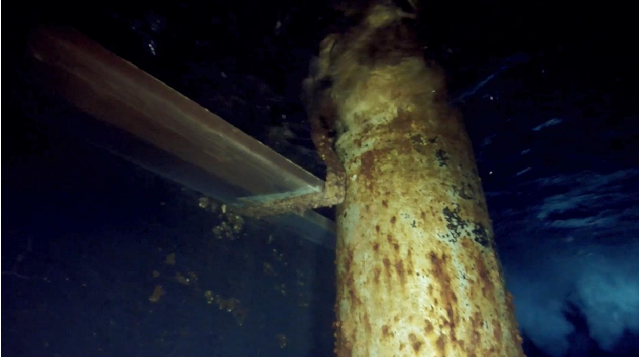
BACKWASH PUMP NO. 3 SUCTION PIPING AT WATER SURFACE
