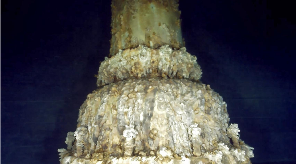
BACKWASH PUMP NO. 3 FOOT VALVE
