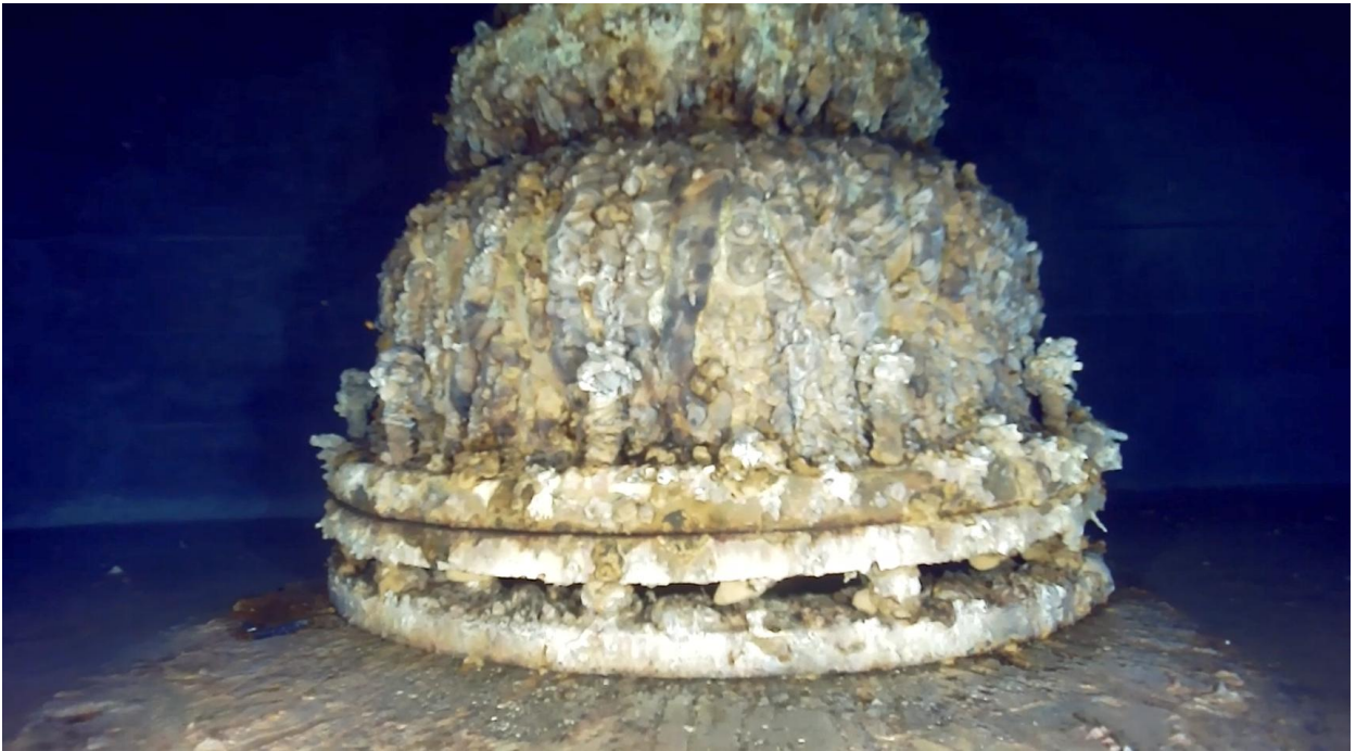
BACKWASH PUMP NO. 3 FOOT VALVE
