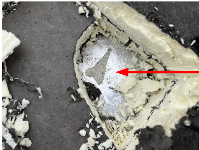
FAN FOIL VAPOR RETARDER THAT NEEDS TO BE REMOVED N.T.S.
